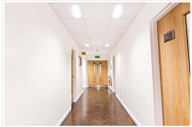
Axant LED installed in a corridor.
