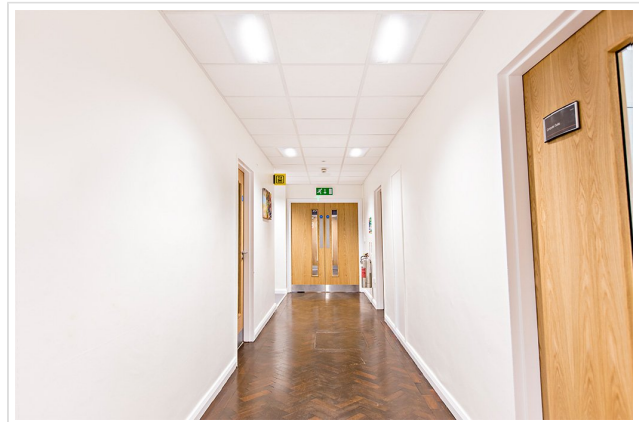
Axant LED installed in a corridor.
